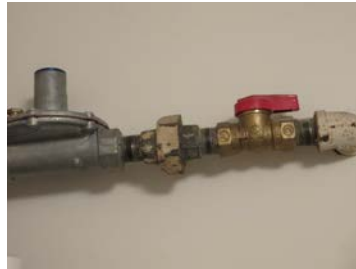
Gas turnoff valve
