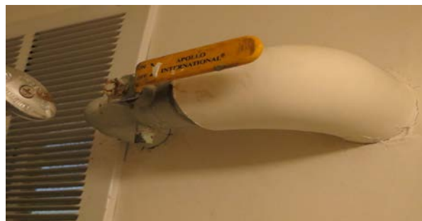
Water turnoff valve
